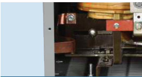
Factory installed main grounding lugs
